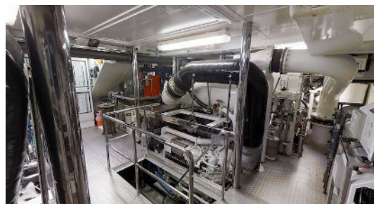
Mechanical Room, Aurora Yacht
